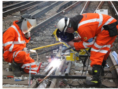
Fig. 4. Rough conditions for track workers © Network Rail UK
